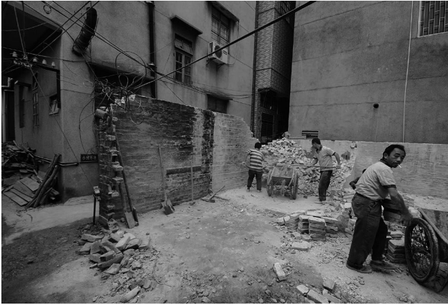
Figure 2: The urban metabolism in operation. Here an older building in Xiaozhoucun is being torn down. The bricks are carefully cleaned of residual mortar, stacked, and stored somewhere nearby for their eventual reuse in the this or another location. The typical new construction is a concrete frame with a single layer of brick used as infill meaning the same material salvaged from a cavity wall masonry structure such as this one can be used to enclose a much larger building. (photo by author)
